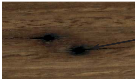
Nail holes, some with tannin staining in nail holes
